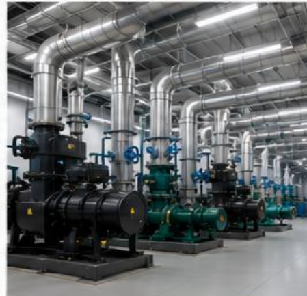
ACMV & MECHANICAL WORKS
