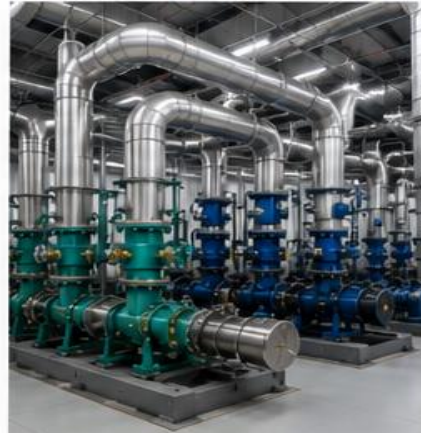
CHILLED WATER PIPING
